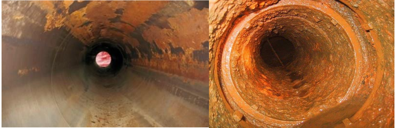
Fig. 2 – Pipes with corrosion
